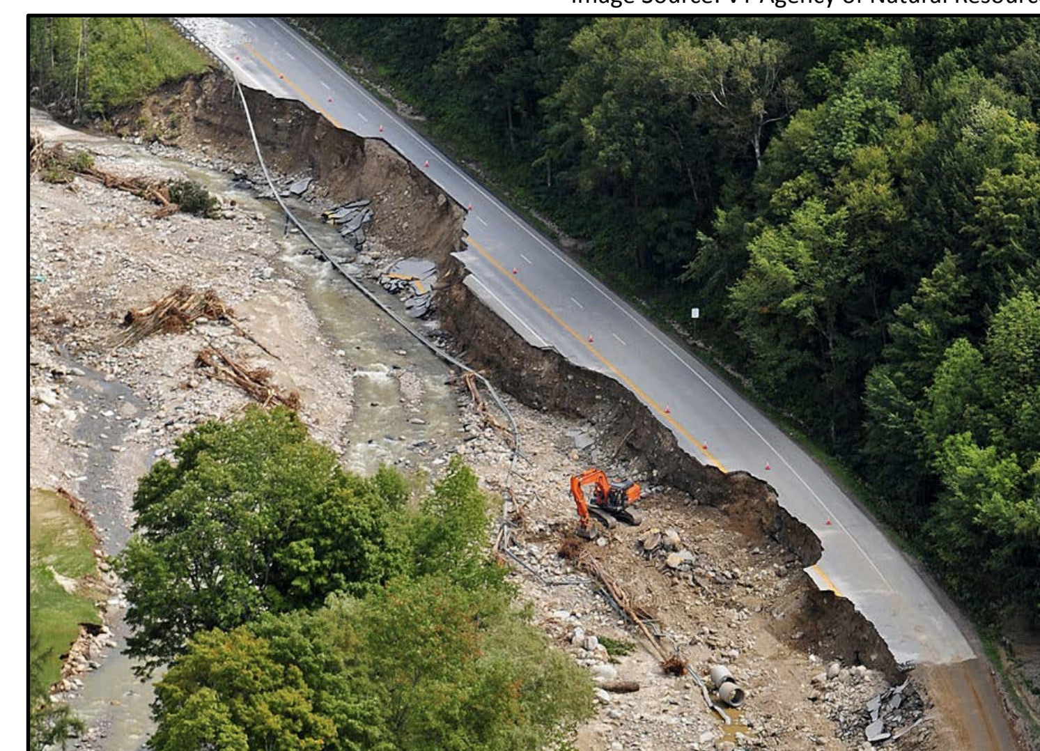
Flooding Damage During Hurricane Irene Image Source: VT Agency of Natural Resources
