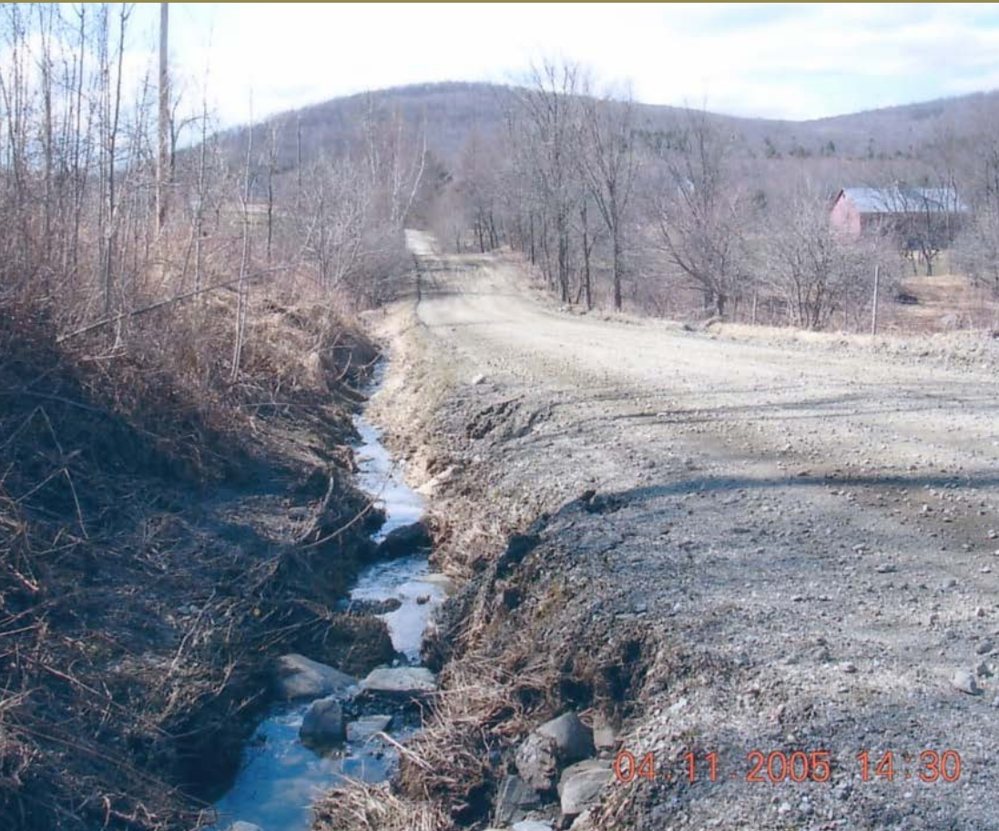
Eroding roadside ditch
