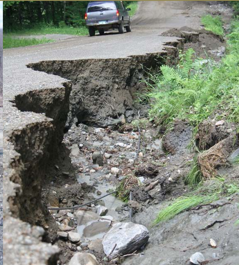
Storm-damaged gravel road
