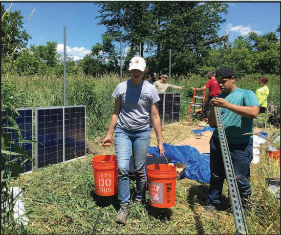
Undergraduate interns Kunal Palawat and Ernesto Vazquez put up solar panels.
